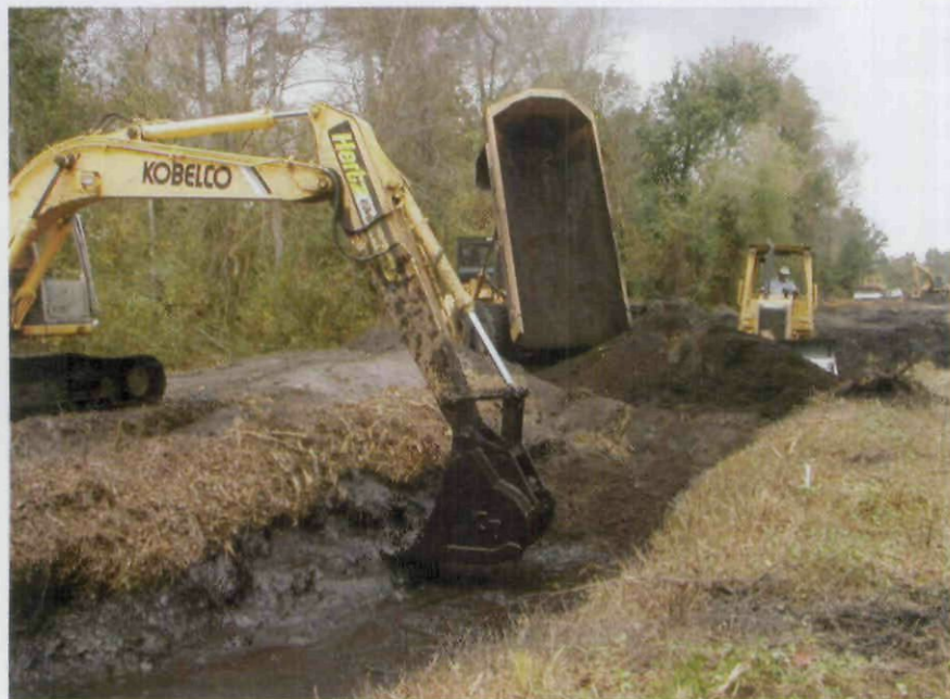
At a mitigation-banking site in North Carolina, workers convert former agricultural land to wetlands. (Photograph courtesy of George Howard, Restoration Systems.)
