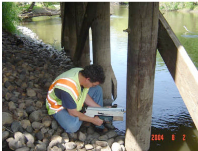
Figure 3. Mn/DOT engineer using a resistance drill to determine the structural condition of a Wright County bridge timber pile.
