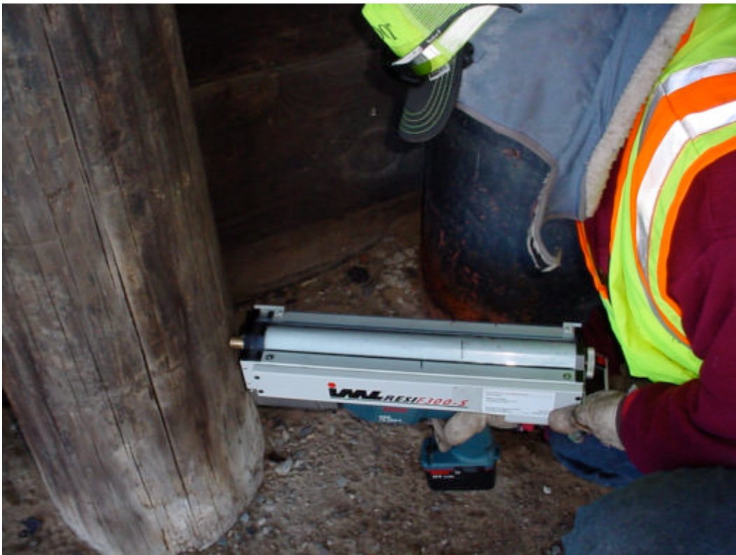
Figure 2. Mn/DOT inspector completing a resistance drill test on a timber piling on bridge 5919.
