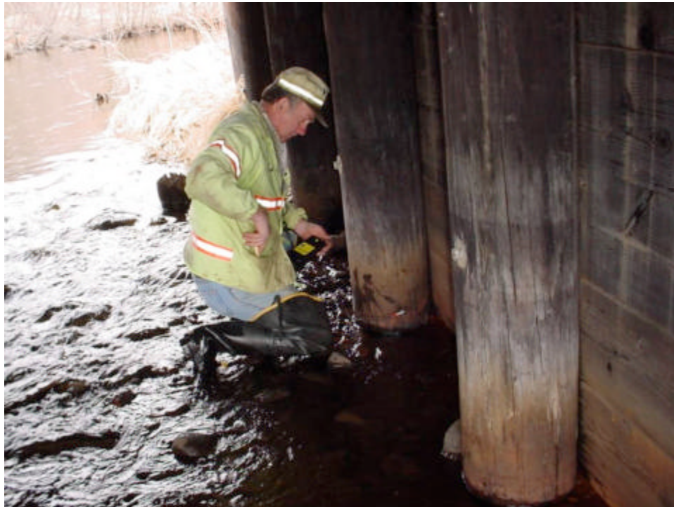
Figure 2. Aitkin County bridge inspector using a Fakopp stress wave timer to assess the structural condition of timber pilings.
