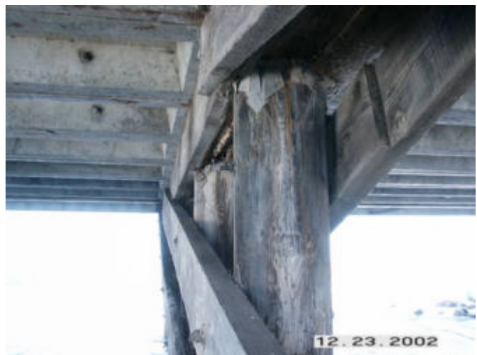
Figure 1. Timber pier cap failure on bridge 56509 in Ottertail County, Minnesota.
