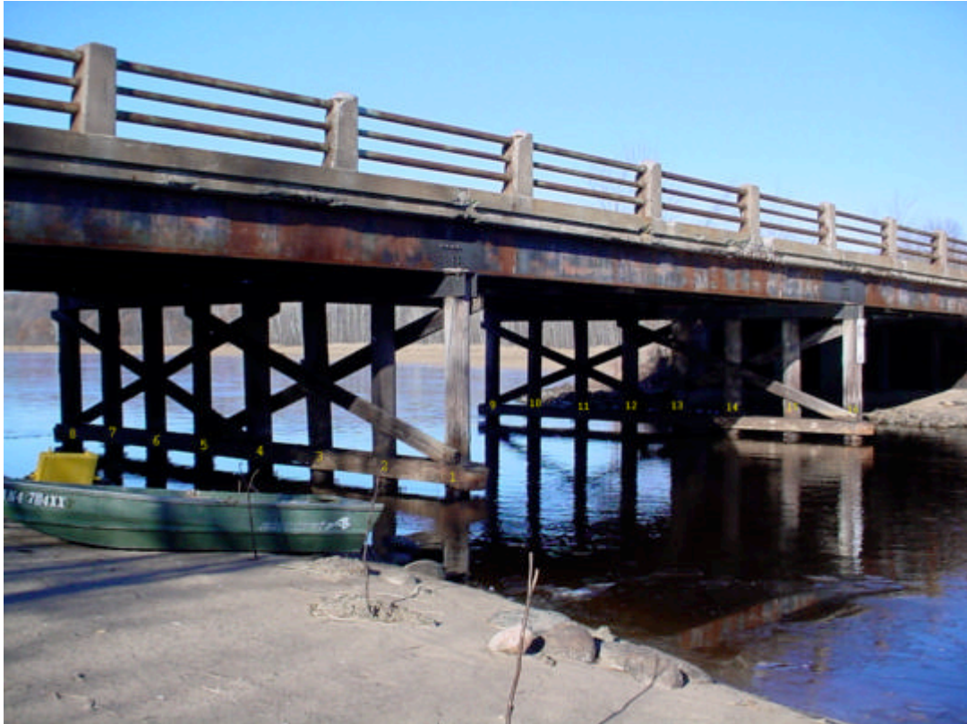
Figure 2. Bridge 5919 showing the 16 timber pilings inspected with a resistance drill 12-18 inches above the waterline.
