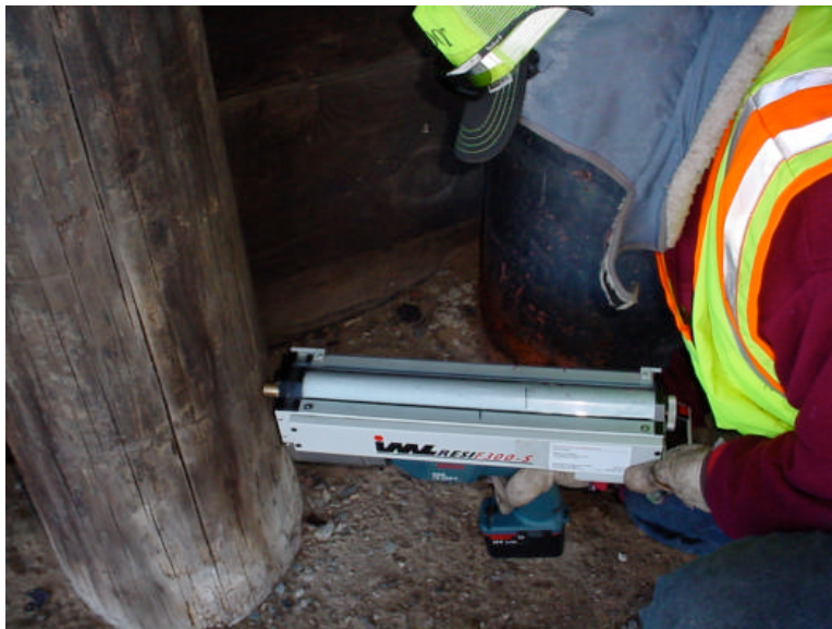
Figure 6. Mn/DOT inspector completing a resistance drill test on a timber piling on bridge 5919.
