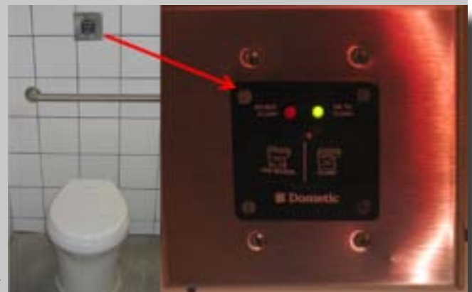
Close-up of the composting toilet flush mechanism
